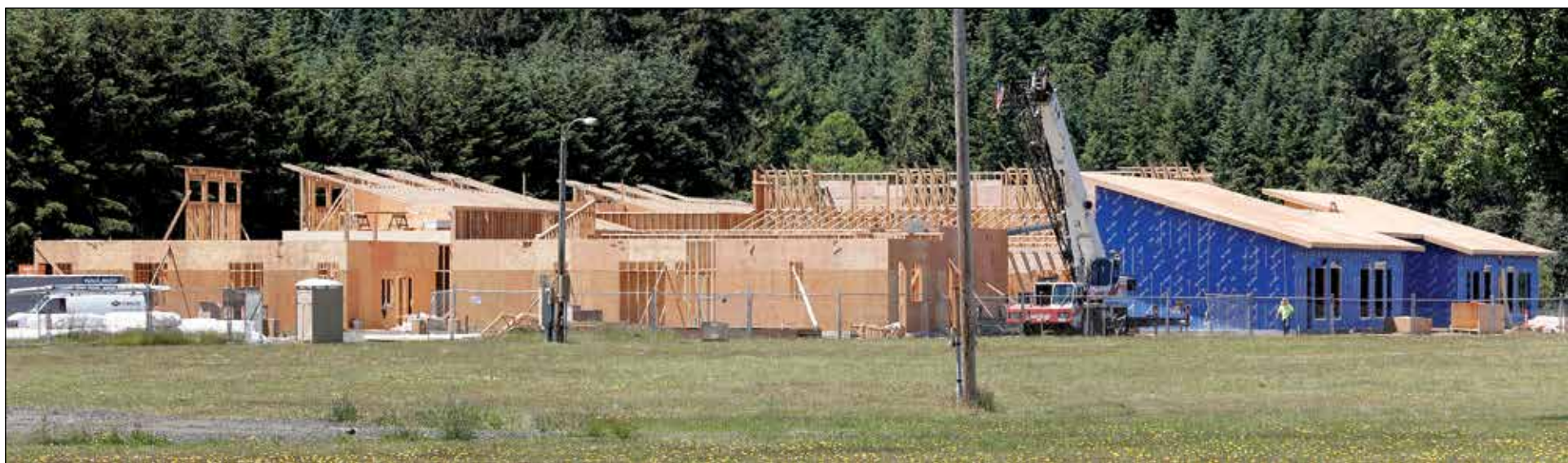
Construction of the 26,000-square-foot child development center began in December 2023 and is expected to be completed in February 2025.
