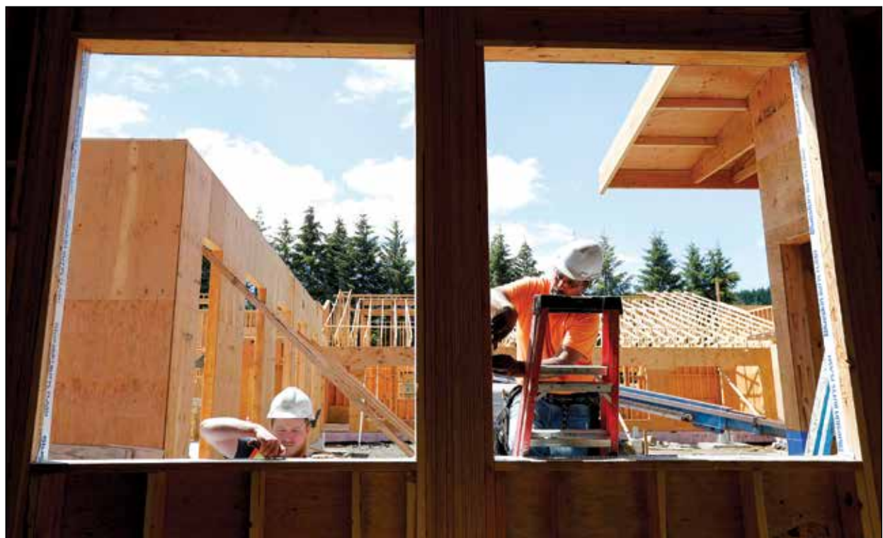
Huri Scherbakob, left, and Javier Mota, both siders with Bold Elements of Woodburn, apply an air, water and moisture vapor barrier to a window while working on the child development center under construction on the Tribal campus on Tuesday, June 18.
