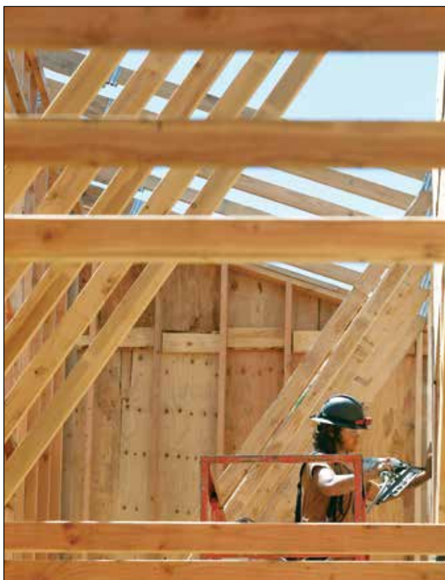
Tribal member Ray Larsen, a carpenter with Triplett Wellman of Woodburn, works on a wall while constructing the child development center.
